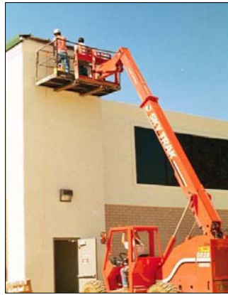
SAFETY WORK PLATFORM
